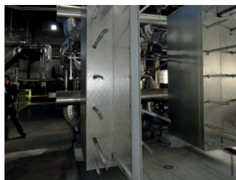
ADP heat exchangers
